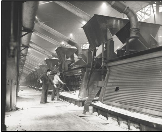
Horizontal Stud Søderberg pots at Tacoma, WA
